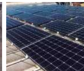
Solar power generation panels at NiGK Corporation
