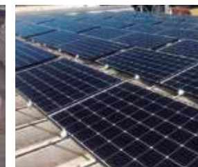
Solar power generation panels at NiGK Corporation
