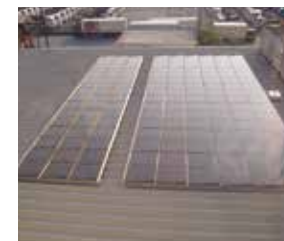
Solar power generation panels at Kawasaki Works
