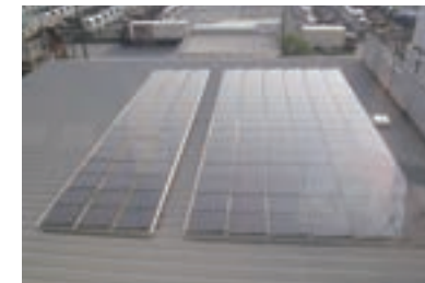
Solar power generation panels
