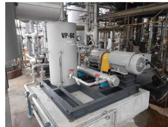
Vacuum pump (Oita Works)
