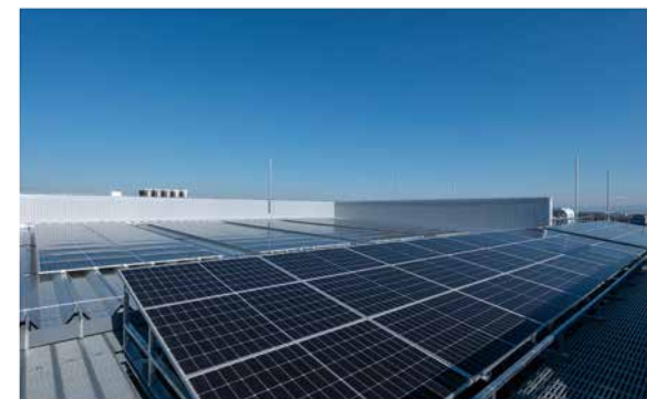
Solar panels at LS Aichi Plant (began operation in April 2025)
