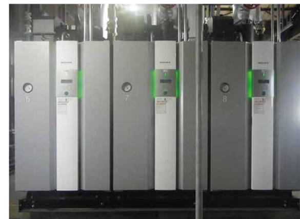
Boiler at the Taketoyo Plant where fuel was converted to city gas (began operating in January 2025)
