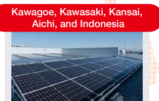
Installed solar panels
