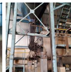
Boiler using biomass fuel
