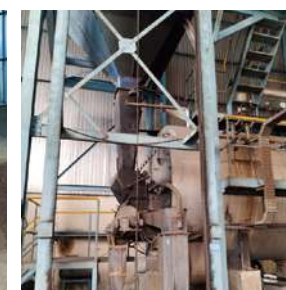
Boiler using biomass fuel
