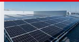
Installed solar panels
