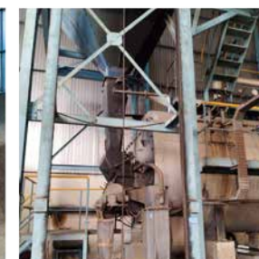
Boiler using biomass fuel
