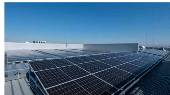
Solar panels at LS Aichi Plant (began operation in April 2025)
