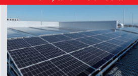
Installed solar panels
