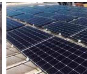
Solar power generation panels at NiGK Corporation
