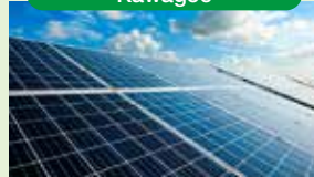
Solar panels (NiGK Corporation)
