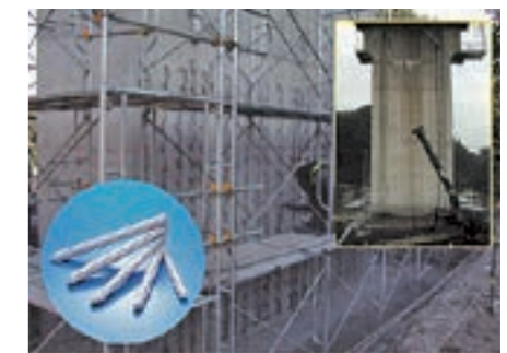
Example of use in an actual project (anti-earthquake reinforcement of Shinkansen bridge piers)
