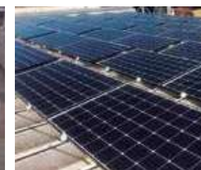
Solar power generation panels at NiGK Corporation
